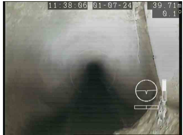
UU MH 4200X_3540daf9-82a2-40d2-940f-2395e0dfdf0f_20240709_152007_796.jpg, 00:02:38, 39.71 m Connection other than junction at 3 o'clock, 450mm dia
