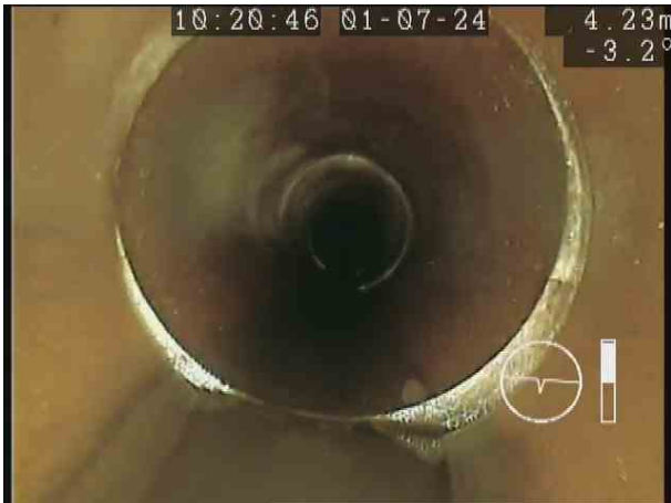
UU MH 5100X_dabed396-6958-49cf-9c10-f389e09b3ef0_20240709_1 61444_292.jpg, 00:00:50, 4.33 m Joint displaced, medium
