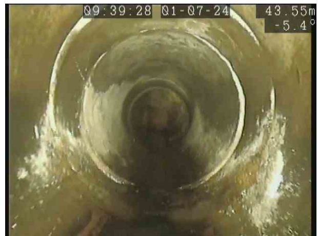
UU MH 6102X_5fa5dfff-6f48-417e-b0eb-d9ced27bb390_20240710_114839_437.jpg, 00:03:06, 43.55 m Crack, circumferential from 9 o'clock to 3 o'clock
