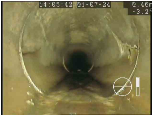
UU MH 7003X_39d22598-ed13-48dd-851e-36eb0247e3a5_20240710_131216_796.jpg, 00:00:22, 0.46 m Crack, longitudinal at joint at 3 o'clock
