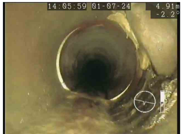
UU MH 7003X_d072b720-dd94-4ec0-b578-884a22fa18aa_20240710_131430_220.jpg, 00:00:39, 4.91 m Connection other than junction at 2 o'clock, 150mm dia
