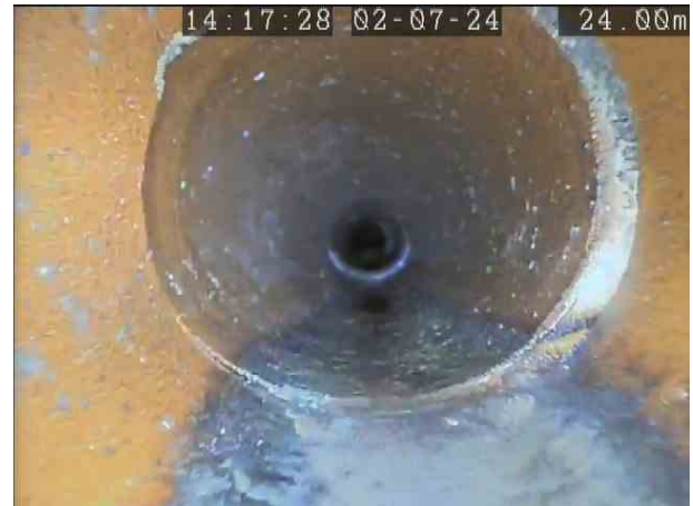
UU MH 6105X_af66cf54-5101-4743-a9e5-3f663224a474_20240710_120736_173.jpg, 00:01:50, 24.00 m Joint displaced, medium
