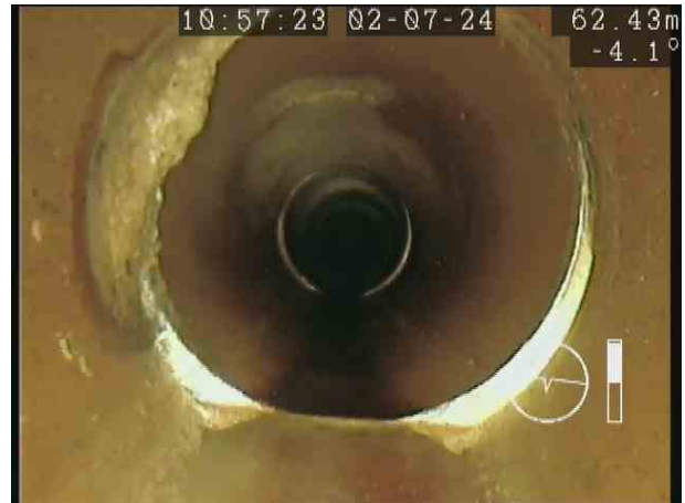
UU MH 5200X_4d6e345a-ce44-4e67-bf9e-cc2b71976528_20240709_165056_494.jpg, 00:04:30, 62.43 m Joint displaced, medium
