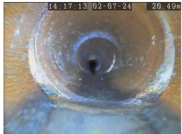
UU MH 6105X_af3257f3-f8b8-428f-b884-add7e31acfee_20240710_120621_025.jpg, 00:01:35, 20.49 m Joint displaced, medium
