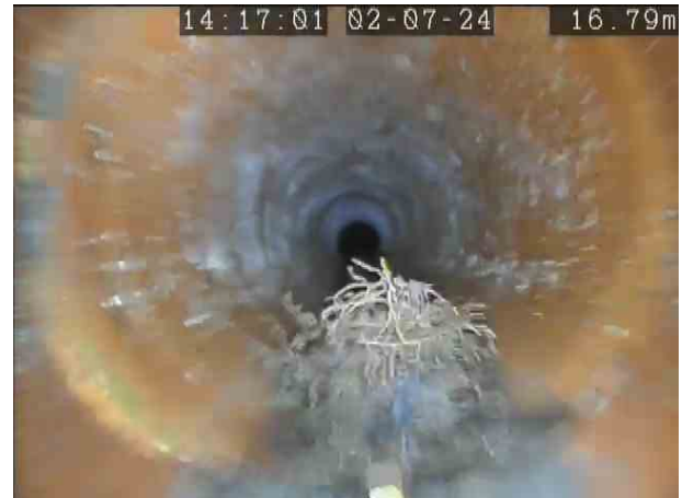
UU MH 6105X_2910cbd9-8aaf-44f8-8c9c-7335619211cf_20240710_120500_273.jpg, 00:01:22, 16.80 m Roots, mass, 10% cross-sectional area loss
