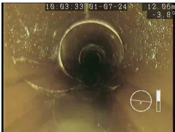
UU MH 6100X_1f1a0399-e9c0-4ff8-963c-9b5585b60a92_20240709_1 61947_196.jpg, 00:01:05, 12.06 m Broken pipe at joint from 5 o'clock to 12 o'clock
