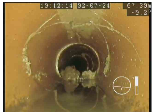
UU MH 6207X_a5faa638-d1eb-480c-9e4c-966253962b1d_20240710_103655_804.jpg, 00:06:37, 67.30 m Cracks, multiple from 9 o'clock to 3 o'clock
