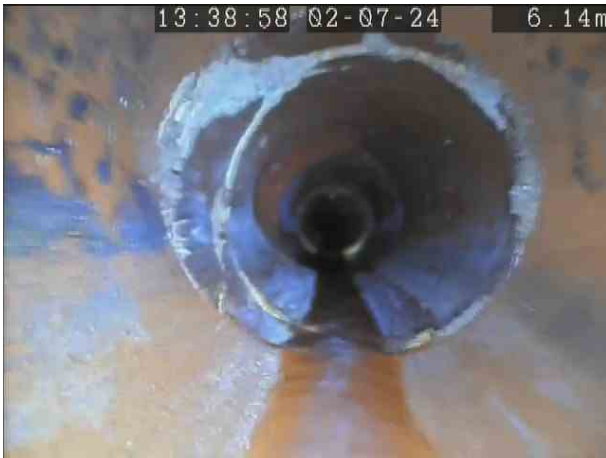
UU MH 5211X_9e05bcb6-a4fe-41b7-afef-8320a649b797_20240710_1 11844_421.jpg, 00:00:34, 6.14 m Cracks, multiple at joint from 7 o'clock to 2 o'clock
