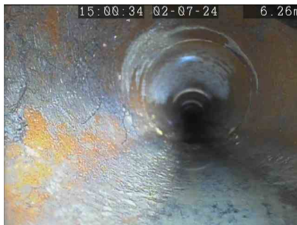
UU MH6107BX_9759681b-13e9-42b2-b4ec-09378cc404ba_2024 0710_125837_465.jpg, 00:00:42, 6.26 m Crack, circumferential at joint from 11 o'clock to 2 o'clock
