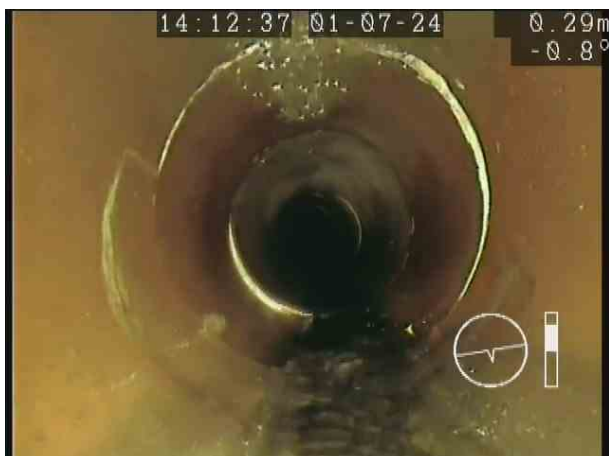
UU MH 7100X_6a00a2a1-d015-41d1-a740-7944b7392f84_20240710_132141_314.jpg, 00:00:14, 0.30 m Crack, circumferential from 12 o'clock to 12 o'clock
