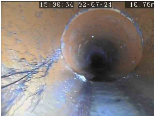
UU MH6107BX_e794da5a-2766-412c-8f4f-52b6a3a5d004_20240 710_125946_733.jpg, 00:01:02, 10.76 m Roots, fine at joint
