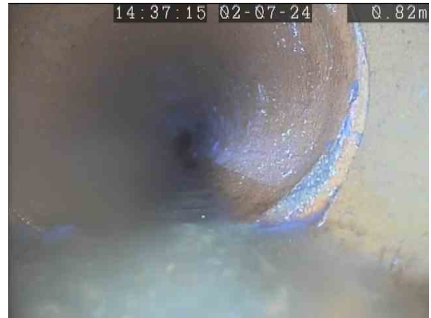
UU MH 6107X_019db6a9-27da-4002-916a-c08b45844871_20240710_121142_782.jpg, 00:00:18, 0.82 m Joint displaced, medium
