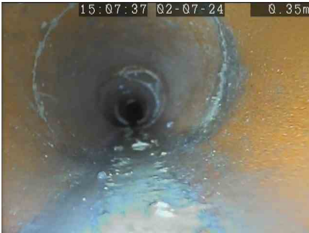
UU MH6107AX_60deeee9-b3ec-49dc-9e27-a0d542f1aef9_20240710_122640_872.jpg, 00:00:18, 0.35 m Crack, circumferential from 8 o'clock to 5 o'clock
