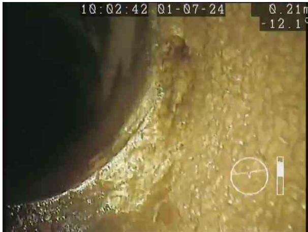
UU MH 6100X_c2b53817-6b05-4afb-a3ce-e00b3135a098_20240709_161749_557.jpg, 00:00:15, 0.21 m Joint displaced, medium
