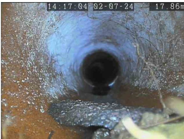
UU MH 6105X_5a17e7c7-ee1c-44d1-ba17-b30ec715055a_20240710_120514_998.jpg, 00:01:26, 17.86 m Settled deposits, coarse, 10% cross-sectional area loss
