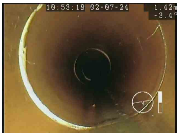
UU MH 5200X_1229c7db-bf6d-4902-bab0-a17b022407d6_20240709_162809_308.jpg, 00:00:24, 1.42 m Crack, longitudinal at joint at 3 o'clock
