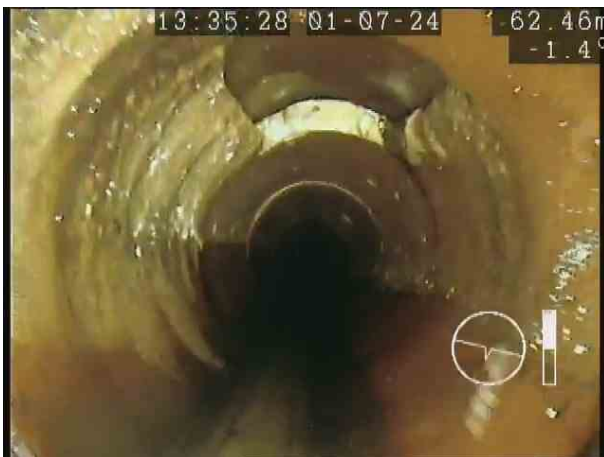
UU MH 6103X_080152c5-dbb7-4dda-96cb-2171be9d353b_20240710_115916_616.jpg, 00:04:10, 62.46 m Hole in drain or sewer from 11 o'clock to 2 o'clock
