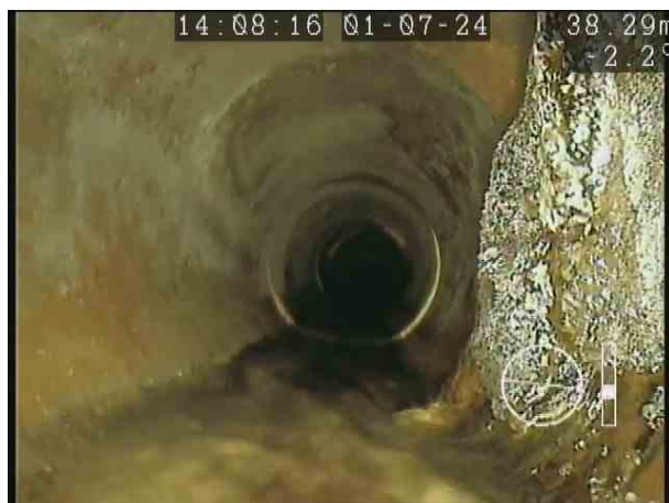
UU MH 7003X_40b91952-7be8-420f-a027-267d743fc8e6_20240710_131821_861.jpg, 00:02:45, 38.29 m Settled deposits, hard or compacted, 25% cross-sectional area loss
