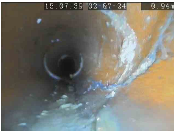
UU MH6107AX_b2cc1fb5-382e-4a3d-8aec-3e866c16732f_20240710_123432_764.jpg, 00:00:19, 0.94 m Fractures, multiple at joint from 8 o'clock to 5 o'clock
