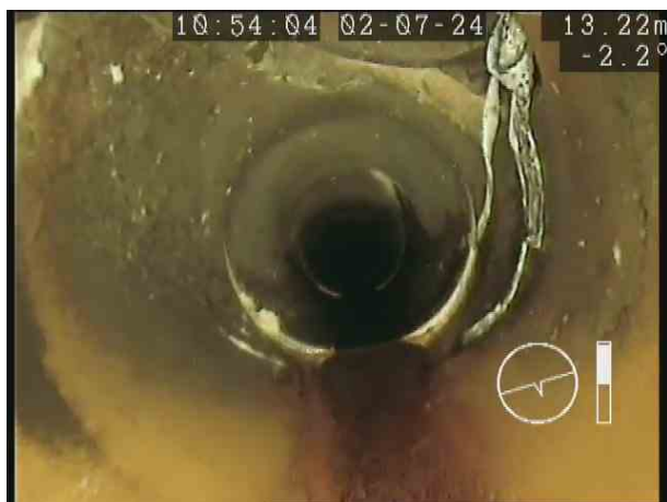
UU MH 5200X_de6db484-6ea8-407a-97d5-1480165ec123_20240709_164347_141.jpg, 00:01:11, 13.22 m Hole in drain or sewer from 12 o'clock to 1 o'clock
