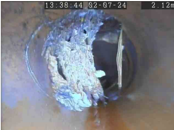
UU MH 5211X_6b865c67-66ec-4510-aacd-cbd0aedc6223_20240710_105654_642.jpg, 00:00:20, 2.12 m Roots, mass, 40% cross-sectional area loss
