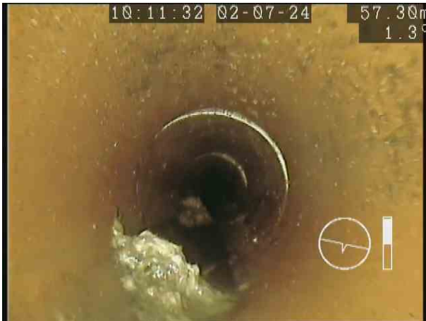
UU MH 6207X_2be9c668-7d39-435e-a14b-870aaf0c4e49_20240710_103223_137.jpg, 00:05:55, 57.30 m Settled deposits, coarse, 10% cross-sectional area loss
