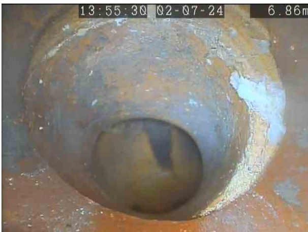
UU MH 5213X_5870cb10-39e8-4fdb-86cd-f072cebb836a_20240710_113657_427.jpg, 00:00:44, 6.86 m Joint displaced, large
