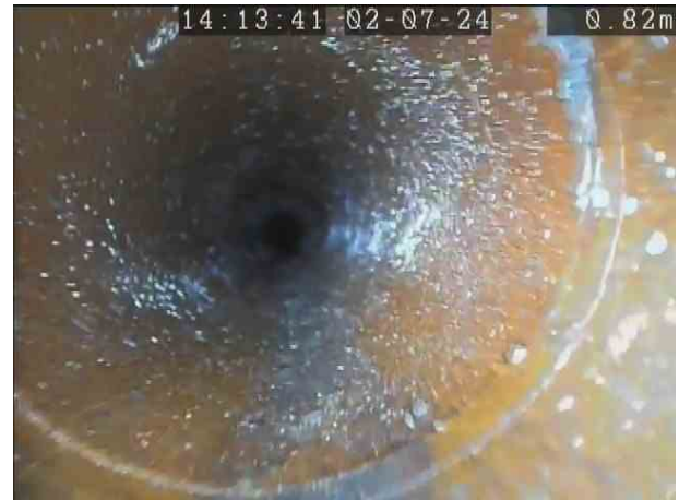
UU MH 6104X_760edf22-034b-4db0-be04-d189a115e6e9_20240710_120912_063.jpg, 00:00:15, 0.82 m Crack, circumferential at joint from 3 o'clock to 6 o'clock
