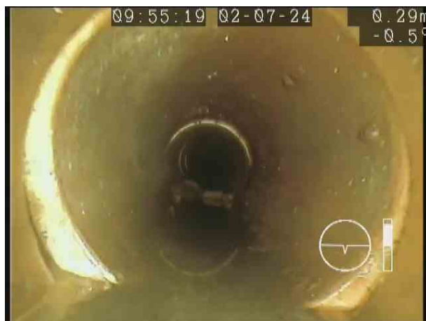
UU MH 6207X_6ac81526-0cc3-4058-9d79-e8525e6cf71f_20240710_102242_608.jpg, 00:00:20, 0.30 m Joint displaced, medium
