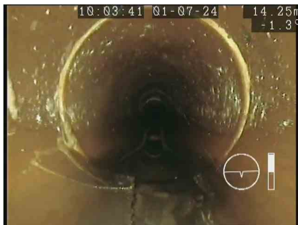
UU MH 6100X_98c78042-5e67-4379-a07d-c180488df7fa_20240709_ 162110_829.jpg, 00:01:12, 13.68 m Broken pipe from 5 o'clock to 1 o'clock
