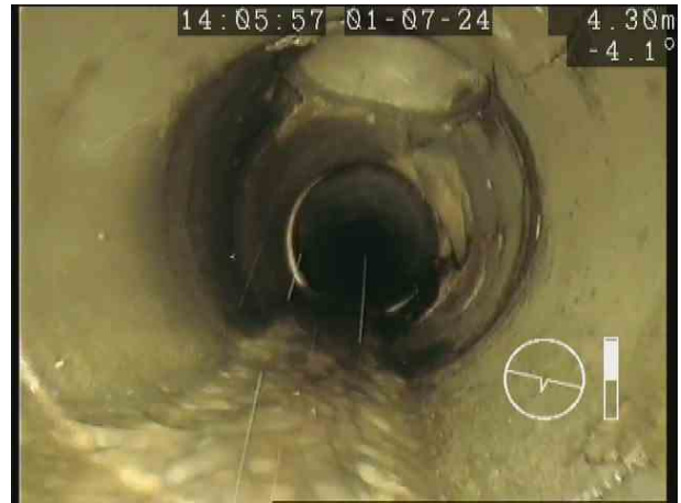
UU MH 7003X_f878f780-b348-436f-9ff8-01ed2215a29e_20240710_131432_748.jpg, 00:00:37, 4.30 m Connection other than junction at 12 o'clock, 100mm dia
