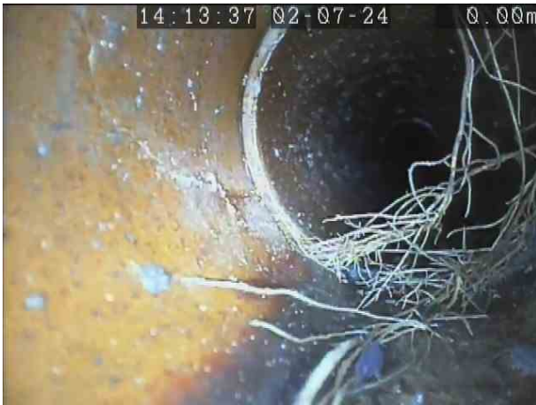
UU MH 6104X_e57cd18b-47aa-4901-9340-26b7bb8bac69_20240710_120853_392.jpg, 00:00:10, 0.05 m Roots, fine at joint
