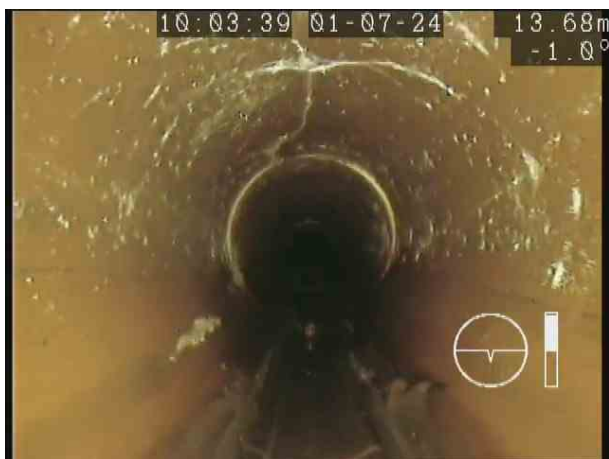
UU MH 6100X_14517ef8-5c0a-41a8-a929-72107e33c6fc_20240709_ 162107_885.jpg, 00:01:12, 13.68 m Broken pipe from 5 o'clock to 1 o'clock
