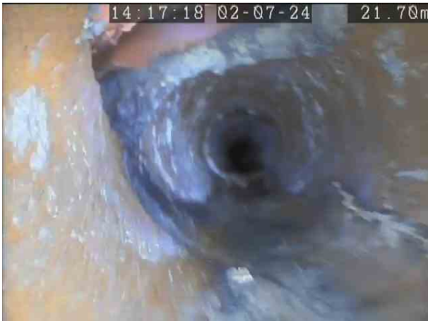
UU MH 6105X_f235f7a2-17e9-461d-b9db-a8749b1bfd16_20240710_120715_846.jpg, 00:01:39, 21.70 m Hole in drain or sewer from 10 o'clock to 11 o'clock
