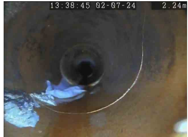
UU MH 5211X_37e35f33-624f-4214-946f-d6d48fcd2c6a_20240710_105726_327.jpg, 00:00:21, 2.24 m Crack, circumferential from 2 o'clock to 7 o'clock
