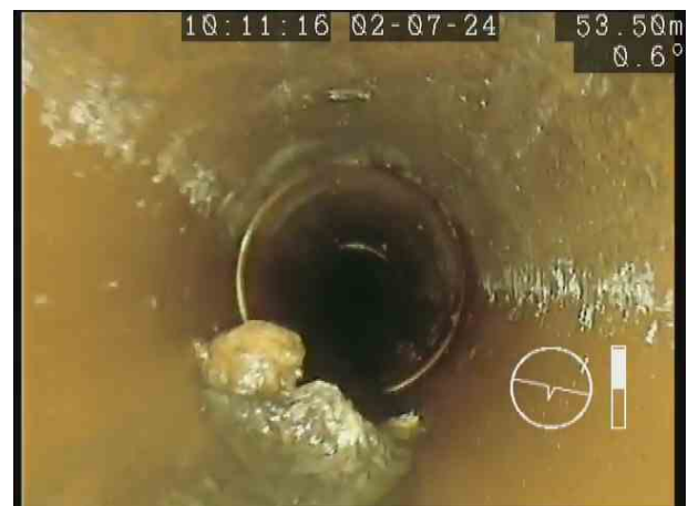
UU MH 6207X_b7cfd917-8e21-465a-ba94-a7a49212c62d_20240710_103154_292.jpg, 00:05:39, 53.50 m Settled deposits, coarse, 10% cross-sectional area loss
