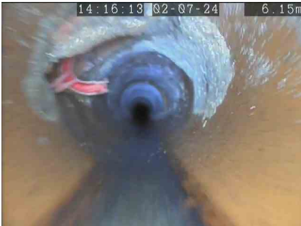
UU MH 6105X_4d1f5dd7-8515-40d9-8cd8-5f252977e062_20240710_120258_758.jpg, 00:00:35, 6.15 m Connection defective, position incorrect at 10 o'clock, 100mm dia
