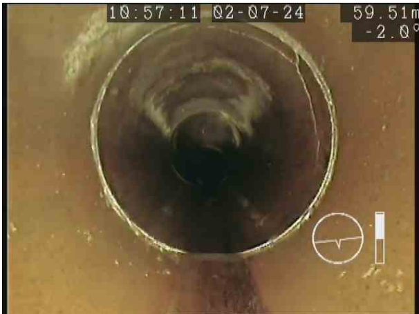
UU MH 5200X_969b0da7-9035-4c91-a55d-c4febf79c8eb_20240709_165040_872.jpg, 00:04:18, 59.51 m Crack, circumferential at joint from 11 o'clock to 4 o'clock
