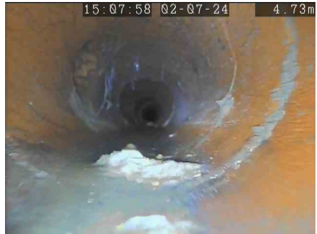
UU MH6107AX_775fc9b6-a6ee-499b-8e54-66e659bd058f_20240710_124000_810.jpg, 00:00:40, 4.73 m Crack, circumferential from 2 o'clock to 5 o'clock
