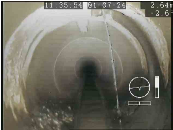
UU MH 4200X_b3b71925-36fc-4632-8215-aaa0aa7d2fc7_20240709_151857_279.jpg, 00:00:25, 2.64 m Connection other than junction at 1 o'clock, 150mm dia
