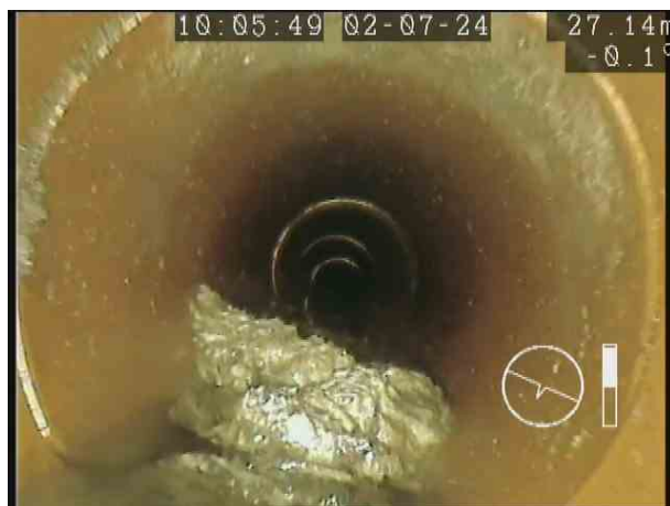
UU MH 6207X_b5834c25-c68b-4485-9ecc-4058e51648b0_20240710_102518_980.jpg, 00:02:27, 27.14 m Settled deposits, coarse, 20% cross-sectional area loss
