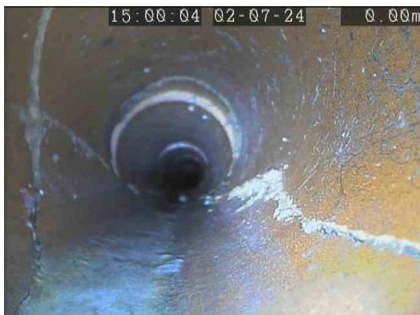
UU MH6107BX_8185fbb7-5422-4a1c-a5e6-f5a7c50f3fd5_202407 10_125314_203.jpg, 00:00:11, 0.01 m Broken pipe from 7 o'clock to 4 o'clock
