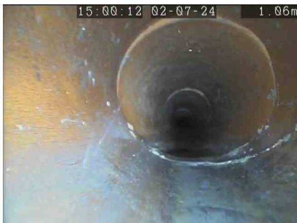
UU MH6107BX_1c4efc2b-4ab0-48ae-9780-c502045f9894_20240 710_125511_877.jpg, 00:00:20, 1.06 m Crack, circumferential at joint from 4 o'clock to 7 o'clock
