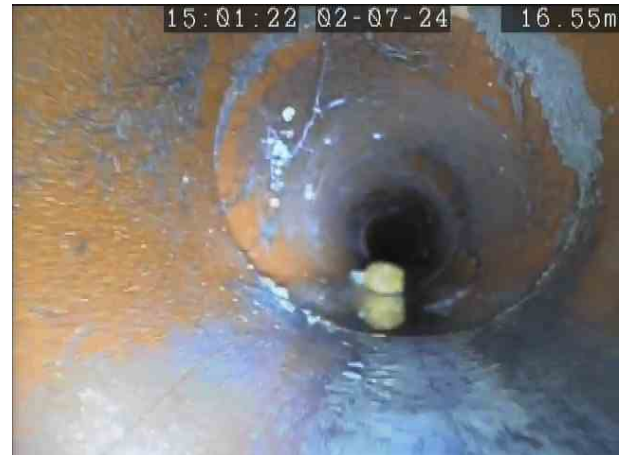
UU MH6107BX_f76e7b26-0422-4fc0-9573-3ca1455930bc_20240 710_130046_218.jpg, 00:01:30, 16.55 m Roots, fine at joint
