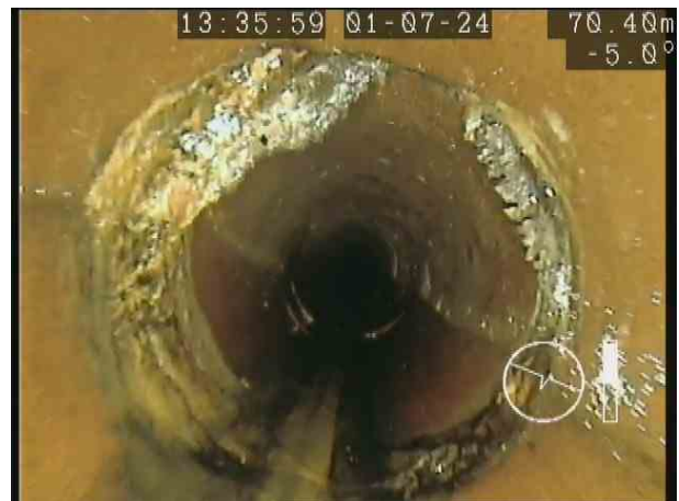
UU MH 6103X_c3cb60a3-84c7-40d5-9167-26202aebd9b6_20240710_115957_714.jpg, 00:04:41, 70.40 m Attached deposits, encrustation at joint from 7 o'clock to 12 o'clock, 15% cross-sectional area loss
