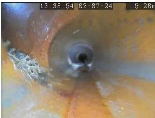
UU MH 5211X_cde71070-dc8f-49d5-b3b3-1298bfbe0920_20240710_105757_292.jpg, 00:00:30, 5.20 m Roots, fine
