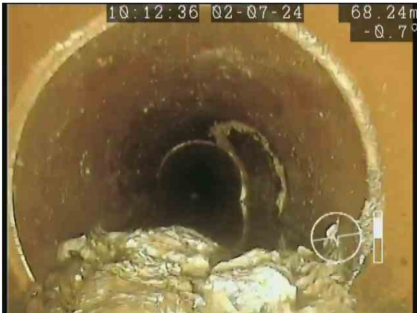
UU MH 6207X_84e34e0f-8c01-41cf-8055-c24d84b8368d_20240710_ 103925_793.jpg, 00:06:59, 68.24 m Settled deposits, hard or compacted at joint, 20% cross-sectional area loss
