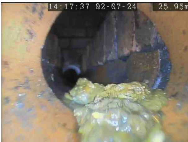
UU MH 6105X_73e42c3a-37ce-435b-846a-90e6df6e0417_20240710_120829_194.jpg, 00:01:58, 25.95 m Settled deposits, other, 20% cross-sectional area loss, Foul waste
