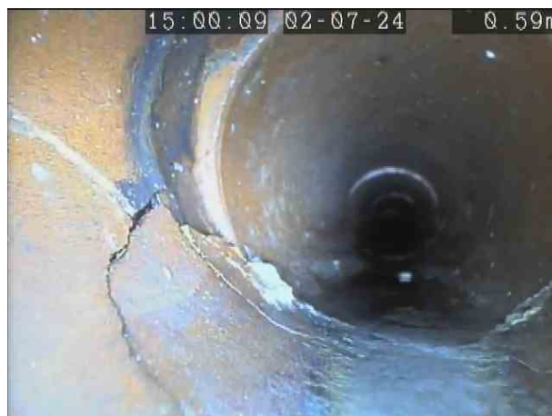
UU MH6107BX_f90ce274-0e12-4431-be83-153d4d29fdcc_20240 710_125427_483.jpg, 00:00:11, 0.01 m Broken pipe from 7 o'clock to 4 o'clock
