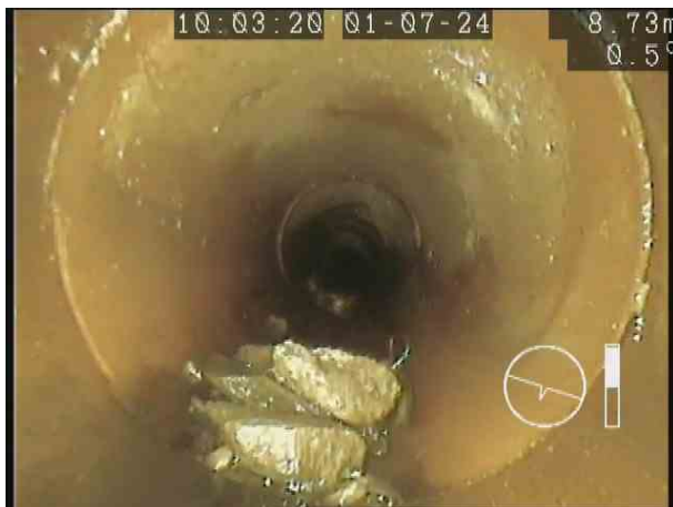
UU MH 6100X_ce0da5d5-0174-49a1-bf84-31fe08bb20a0_20240709_161858_455.jpg, 00:00:52, 8.73 m Settled deposits, coarse, 10% cross-sectional area loss
