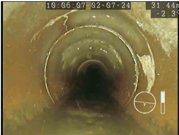
UU MH 6207X_27a63495-2bd2-4348-95e8-6975caa3cb4f_20240710_102819_692.jpg, 00:02:45, 31.44 m Crack, circumferential from 10 o'clock to 4 o'clock
