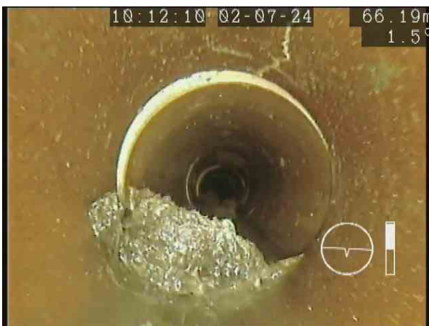
UU MH 6207X_b3f5de73-a7ab-4c17-94dd-ee1b554ca530_20240710_103633_998.jpg, 00:06:33, 66.19 m Settled deposits, coarse at joint, 25% cross-sectional area loss
