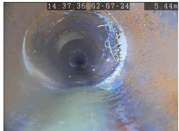
UU MH 6107X_43ef54ee-6462-4dd3-9629-f2ae5a6e2ad0_20240710_121301_321.jpg, 00:00:39, 5.44 m Joint displaced, medium
