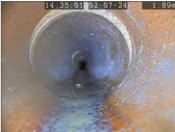
UU MH 6106X_1fecc75b-9457-45b5-87be-956a8c22c349_20240710_121652_147.jpg, 00:00:21, 1.90 m Joint displaced, medium
