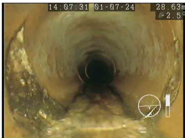
UU MH 7003X_9b082942-0be2-48c7-b25c-257c7d28bdec_20240710_131711_603.jpg, 00:02:11, 28.63 m Attached deposits, encrustation at joint from 7 o'clock to 10 o'clock, 10% cross-sectional area loss
