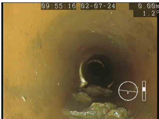
UU MH 6207X_bb3f1c9c-5d26-4bc6-9104-c0a514c6bf04_20240710_102232_924.jpg, 00:00:18, 0.05 m Settled deposits, coarse, 5% cross-sectional area loss
