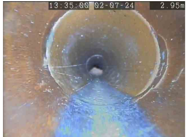
UTPX_49d29612-f96e-424b-bc3e-f3279f944a80_20240710_105417_702.jpg, 00:00:24, 2.95 m Crack, circumferential at joint from 3 o'clock to 6 o'clock
