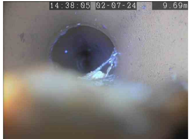
UU MH 6107X_83a80ebc-aa1a-4e04-a946-016255bec334_20240710_121539_392.jpg, 00:01:09, 9.70 m Roots, fine at joint
