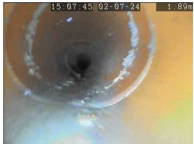
UU MH6107AX_05090492-b964-4d08-a526-19632702de53_20240710_123512_218.jpg, 00:00:27, 1.90 m Crack, circumferential at joint from 8 o'clock to 4 o'clock
