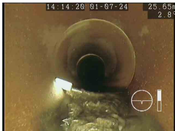
UU MH 7100X_c7d91596-d8b9-48ad-a7f8-5a4550dc115c_20240710_132254_026.jpg, 00:01:56, 25.65 m Settled deposits, hard or compacted, 5% cross-sectional area loss
