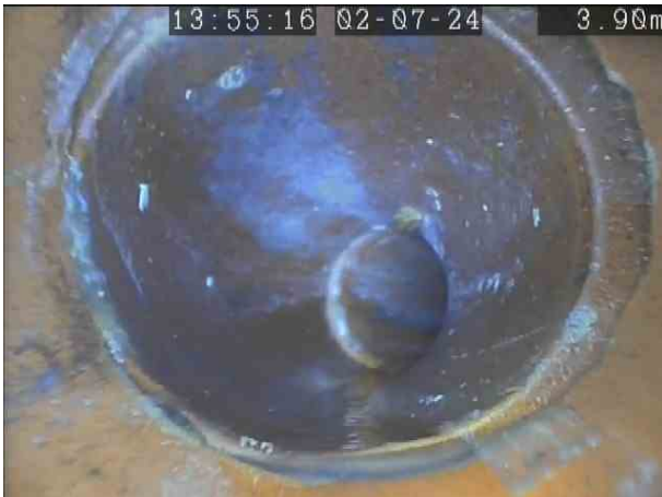
UU MH 5213X_64931727-b749-4265-b018-498b5aff5b9e_20240710_113559_729.jpg, 00:00:29, 3.90 m Open joint, medium
