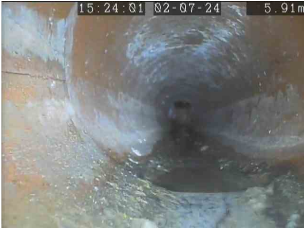
UU MH6107DX_0d254413-0e0f-4d09-9a84-87e98e0450d8_2024 0710_131915_828.jpg, 00:00:34, 5.91 m Crack, longitudinal at joint at 9 o'clock
