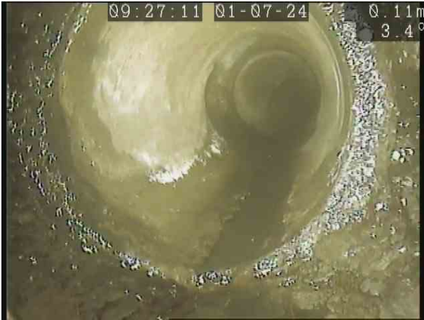
GullyX_c0fb68e5-ac3c-4848-a10f-fa8c97e055ed_20240710_1 14921_945.jpg, 00:00:32, 0.11 m Joint displaced, medium
