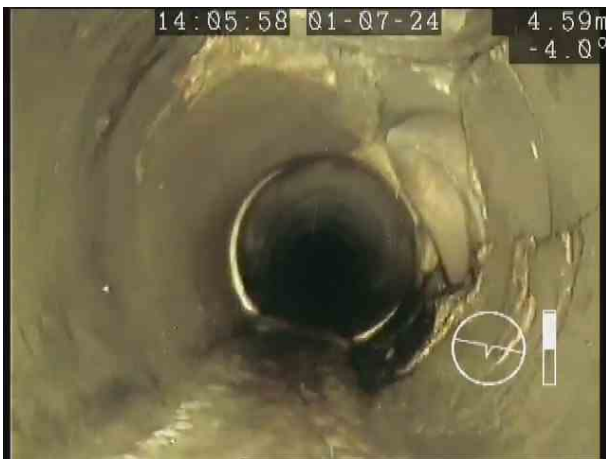
UU MH 7003X_21045095-d4f2-4fdc-ba61-c9b5a75b6702_20240710_131251_216.jpg, 00:00:38, 4.60 m Cracks, multiple from 1 o'clock to 5 o'clock
