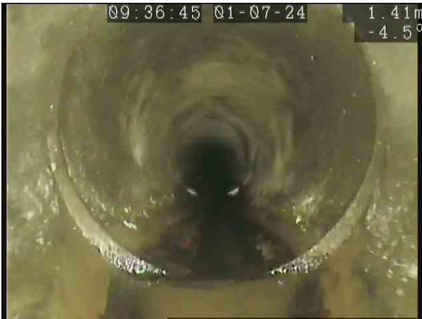
UU MH 6102X_210052a5-baf9-4066-87cf-7e52002475c0_20240710_114315_826.jpg, 00:00:23, 1.41 m Joint displaced, medium
