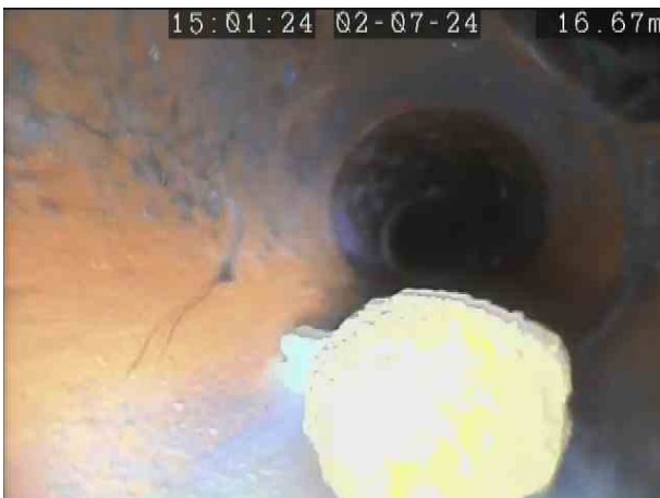
UU MH6107BX_f56d6128-7288-4543-869d-5a95a737b1ef_20240 710_130128_747.jpg, 00:01:32, 16.67 m Settled deposits, other, 10% cross-sectional area loss, Foul waste
