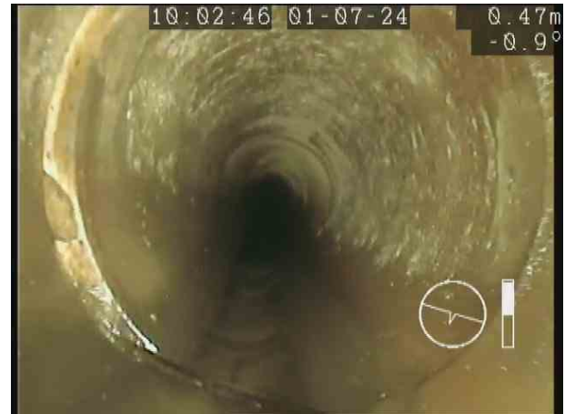
UU MH 6100X_06f56600-acb1-4600-853b-23f0074acdaa_20240709_161808_803.jpg, 00:00:19, 0.47 m Joint displaced, medium
