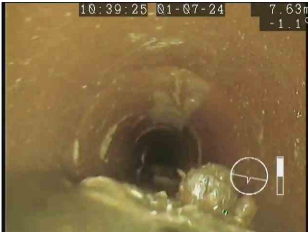
UU MH 6207X_063d7feb-b4c6-43bc-8059-3273d38f87fd_20240710_130802_697.jpg, 00:00:46, 7.63 m Settled deposits, hard or compacted, 25% cross-sectional area loss
