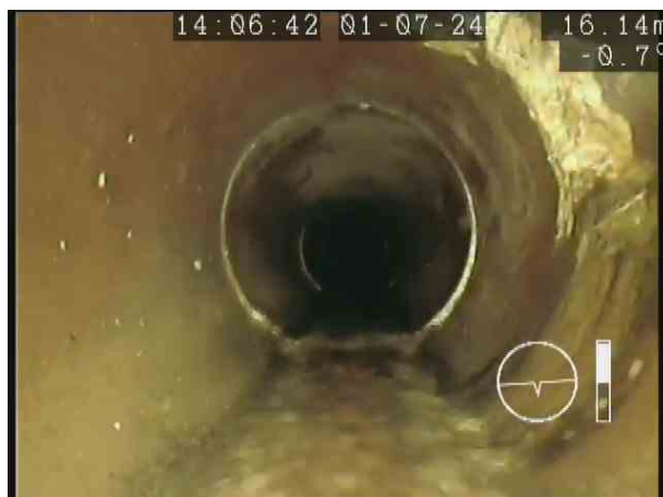
UU MH 7003X_f044fae5-85bc-4edc-82ed-dc73e9bd882b_20240710_131629_982.jpg, 00:01:22, 16.14 m Connection other than junction at 2 o'clock, 100mm dia
