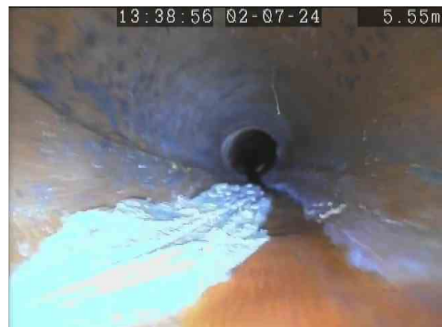
UU MH 5211X_3ef15740-ad7b-4ea4-bd8b-1a8d4dc86e17_20240710_111813_767.jpg, 00:00:32, 5.55 m Settled deposits, other, 5% cross-sectional area loss, Wipe
