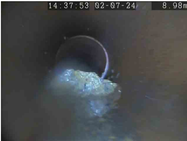
UU MH 6107X_e9d9c869-a0fd-4339-8594-b4829b612499_20240710_121508_481.jpg, 00:00:50, 8.98 m Settled deposits, other, 20% cross-sectional area loss, Debris, being pushed down line by camera
