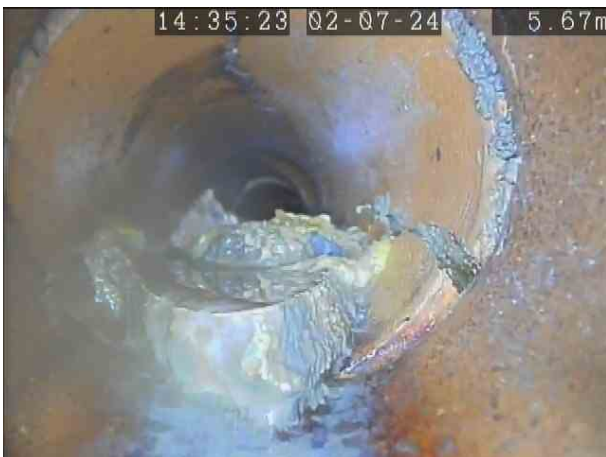
UU MH 6106X_57b8d791-92cf-455c-ada4-c0295a4073fb_20240710_121757_623.jpg, 00:00:43, 5.67 m Broken pipe at joint from 12 o'clock to 4 o'clock
