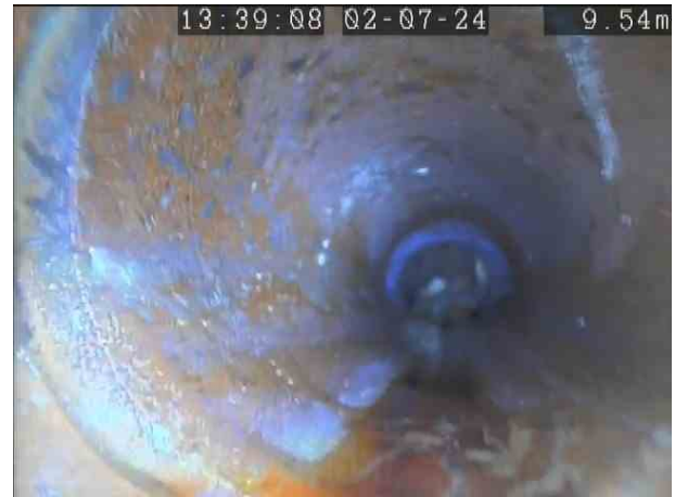
UU MH 5211X_7b511660-2d8d-4962-9f5b-bf9645c94f94_20240710_1 12129_465.jpg, 00:00:44, 9.54 m Open joint, medium
