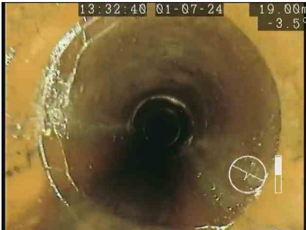
UU MH 6103X_ad477bb1-3347-4377-926c-b51cec39dc9f_20240710_115331_218.jpg, 00:01:23, 19.00 m Crack, circumferential at joint from 5 o'clock to 11 o'clock
