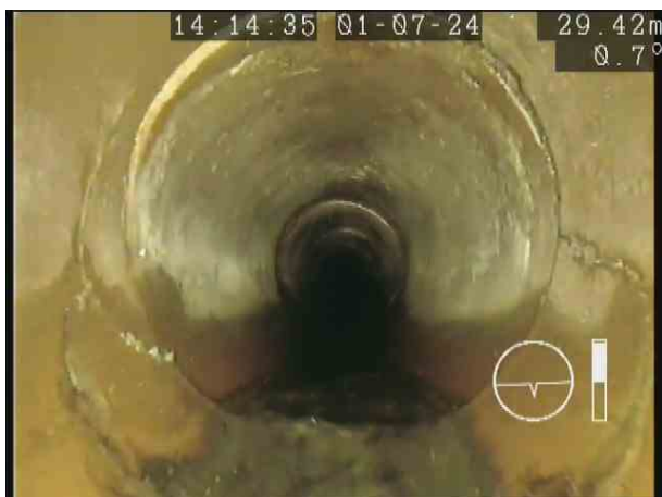
UU MH 7100X_1db507ad-ea16-471e-9689-70e550d0655c_20240710_132319_673.jpg, 00:02:12, 29.42 m Crack, circumferential at joint from 3 o'clock to 10 o'clock
