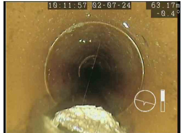
UU MH 6207X_f921eaf1-a966-4dae-b781-45c95009adb5_20240710_103554_089.jpg, 00:06:20, 63.17 m Settled deposits, coarse, 10% cross-sectional area loss
