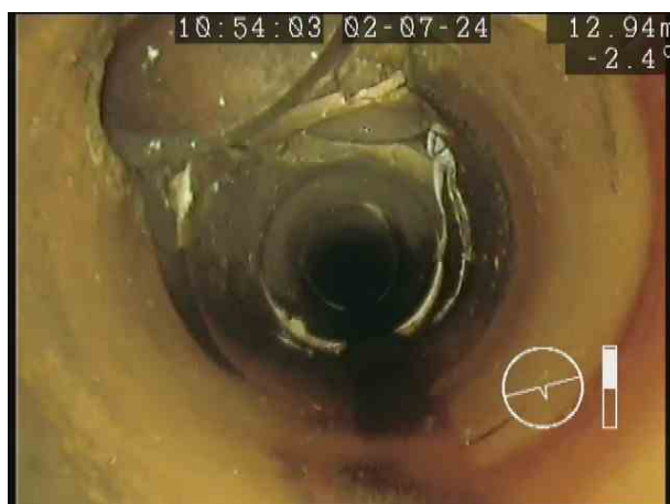
UU MH 5200X_6efc9d5e-2a46-4cac-9093-989770bcc7cf_20240709_164319_582.jpg, 00:01:10, 12.94 m Hole in drain or sewer from 11 o'clock to 12 o'clock
