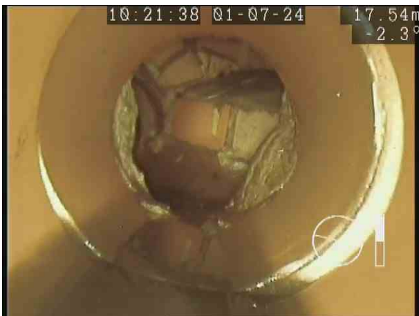
UU MH 5100X_c785e845-9a03-41d0-b460-df0419c3a2c5_20240709_ 161610_181.jpg, 00:01:41, 17.54 m Joint displaced, medium
