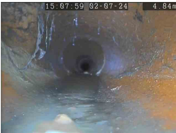
UU MH6107AX_fdf360c8-c7a8-4766-87ac-a77218163a15_20240710_124014_117.jpg, 00:00:41, 4.84 m Roots, fine
