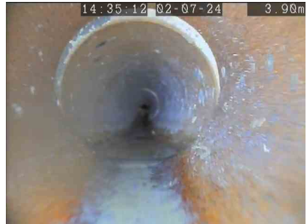
UU MH 6106X_d6ad702c-0bcb-4aa7-8963-6140e1f2550a_20240710_121719_714.jpg, 00:00:31, 3.90 m Joint displaced, medium
