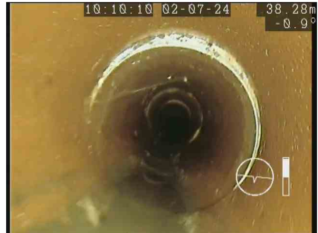
UU MH 6207X_50d6488d-6145-42a9-90f6-950ad5a2d924_20240710_103033_058.jpg, 00:04:33, 38.28 m Joint displaced, medium
