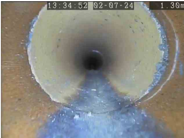
UTPX_4f8e55af-1345-4262-9642-64bc344ad2c4_20240710_105337_545.jpg, 00:00:17, 1.30 m Crack, circumferential at joint from 2 o'clock to 6 o'clock
