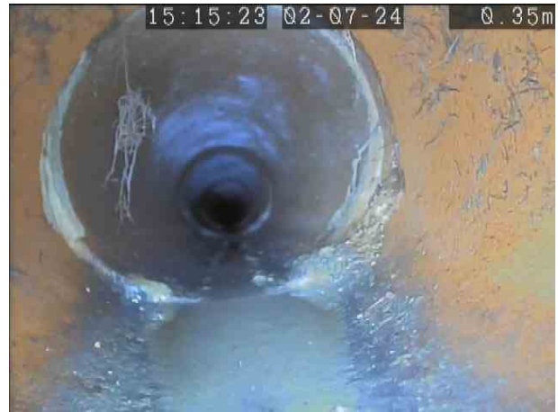
UU MH6107CX_ea0ddb5-7f23-4228-8dc1-2eb74ff659b8_20240 710_130347_264.jpg, 00:00:15, 0.35 m Roots, fine at joint
