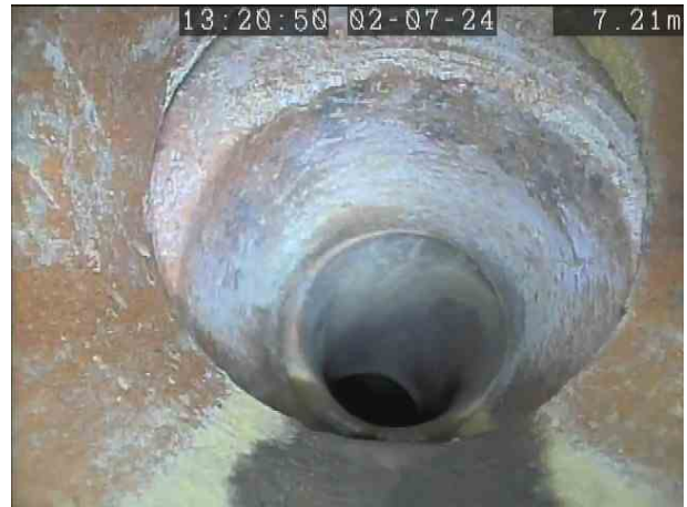
UU MH 4115X_fe222fd2-3392-42d1-b9a6-f58d2eb831c8_20240709_1 50559_290.jpg, 00:00:37, 7.21 m Joint displaced, large
