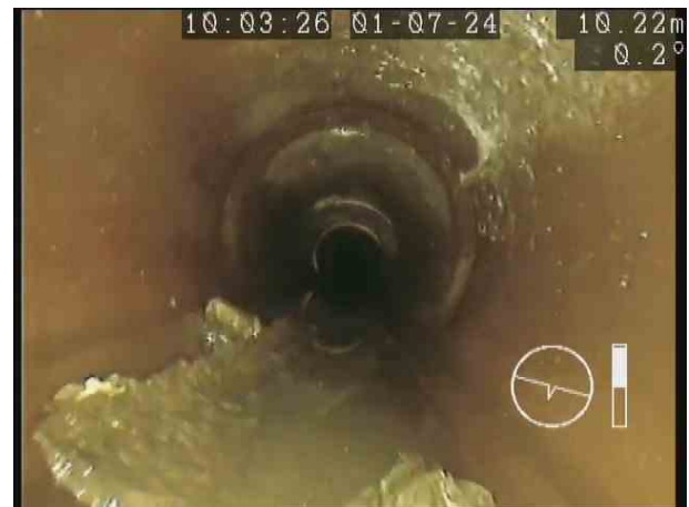
UU MH 6100X_75dea4a6-2fd7-41bb-95b7-5ea55af680c4_20240709_161919_149.jpg, 00:00:58, 10.22 m Settled deposits, hard or compacted, 10% cross-sectional area loss
