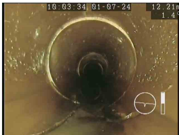
UU MH 6100X_a692a75b-395e-47d1-98bd-1d2c88121c61_20240709 _161949_595.jpg, 00:01:05, 12.06 m Broken pipe at joint from 5 o'clock to 12 o'clock
