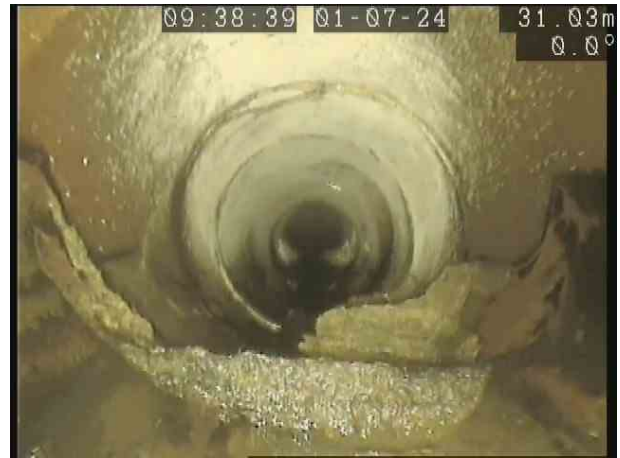
UU MH 6102X_054b9233-0eb6-4d59-b32b-33d4f6c33e59_20240710_114500_483.jpg, 00:02:16, 31.03 m Settled deposits, hard or compacted, 15% cross-sectional area loss
