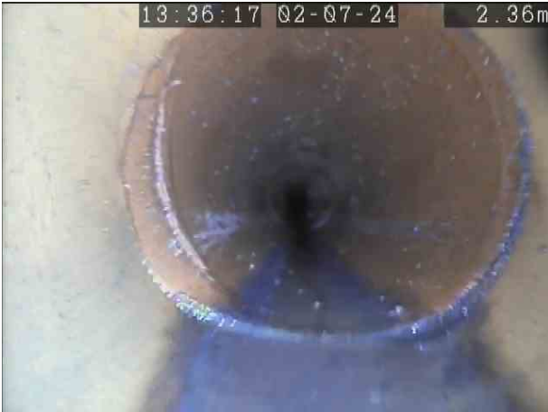
UU MH 5210X_3f16972f-4912-46c5-8064-85a6e59f52ba_20240710_1 05133_216.jpg, 00:00:18, 2.36 m Crack, circumferential from 7 o'clock to 10 o'clock
