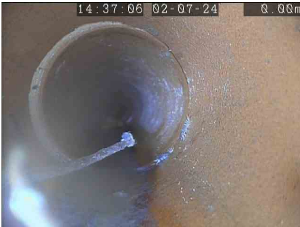
UU MH 6107X_fd70e5fa-89cf-406f-92d8-bbf87f1bf373_20240710_12128_447.jpg, 00:00:10, 0.01 m Roots, tap
