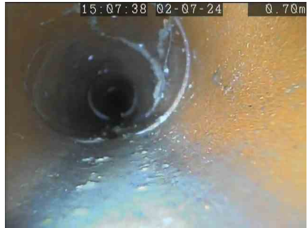
UU MH6107AX_4a8c7710-511d-4ea7-817a-04986cc7a9de_20240710_123428_172.jpg, 00:00:19, 0.94 m Fractures, multiple at joint from 8 o'clock to 5 o'clock
