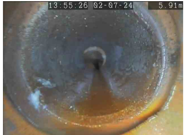
UU MH 5213X_228e18da-f298-4bd3-8efa-29967bba6145_20240710_113639_796.jpg, 00:00:40, 5.91 m Open joint, medium
