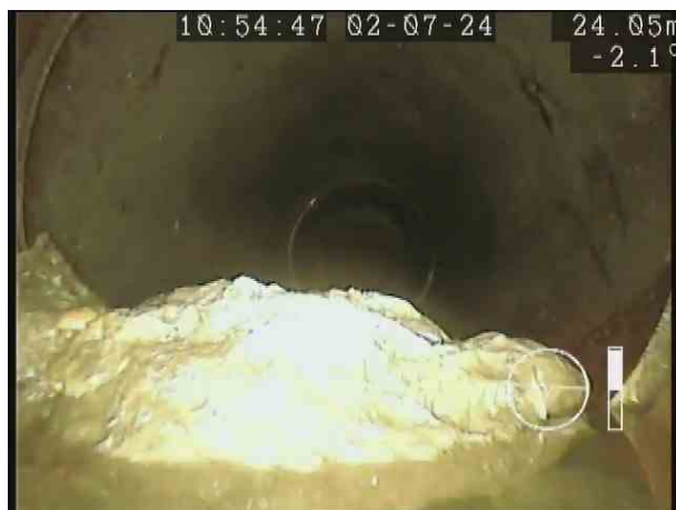
UU MH 5200X_6f434d05-9c17-40f0-8d80-bfeef4df2417_20240709_164854_279.jpg, 00:01:54, 24.05 m Settled deposits, other at joint, 20% cross-sectional area loss, Build of silt/ tissues
