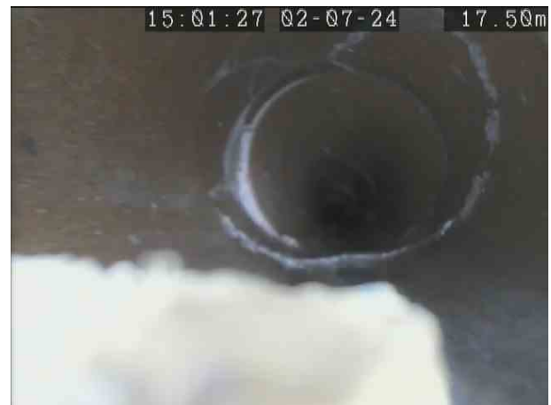
UU MH6107BX_5c05207c-31cc-4b04-85c6-74e607bf22b7_20240 710_130154_126.jpg, 00:01:35, 17.50 m Fracture, circumferential at joint from 12 o'clock to 12 o'clock
