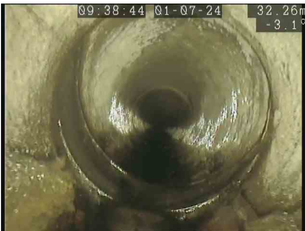
UU MH 6102X_8aa0c46d-9a96-4dd7-baeb-a9c16474a47f_20240710_114547_387.jpg, 00:02:22, 32.26 m Crack, circumferential at joint from 4 o'clock to 10 o'clock
