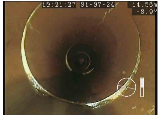
UU MH 5100X_aaf636f2-5770-42cd-81d5-3cd541612f48_20240709_1 61535_640.jpg, 00:01:30, 14.56 m Crack, longitudinal at joint at 1 o'clock
