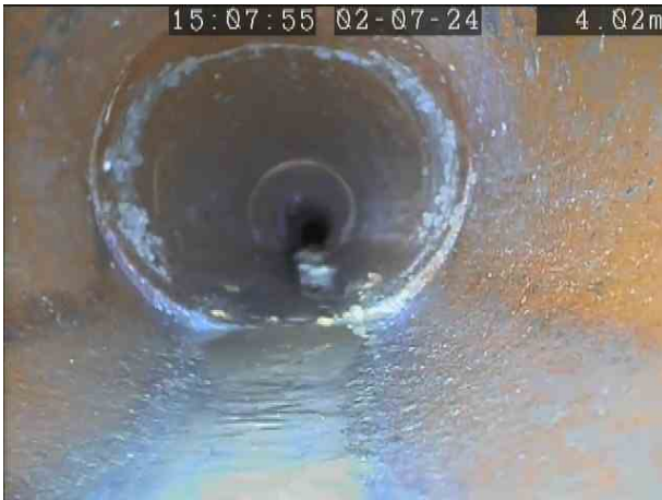
UU MH6107AX_eebef5a0-0d76-464a-8169-e5fea1051d21_20240710_123858_044.jpg, 00:00:36, 4.02 m Crack, circumferential at joint from 8 o'clock to 5 o'clock
