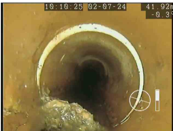
UU MH 6207X_57088977-9eb4-45b4-9e67-b9a661a7ae5f_20240710_103102_897.jpg, 00:04:49, 41.92 m Settled deposits, coarse at joint, 10% cross-sectional area loss
