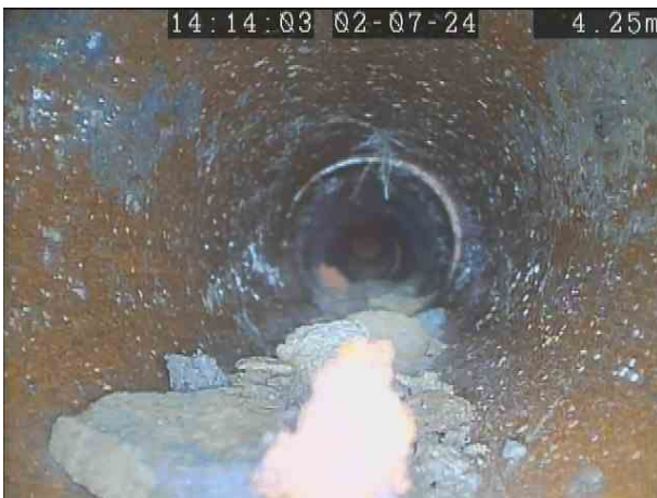
UU MH 6104X_8f393437-a3a7-421d-8605-f4f3c697f217_20240710_120952_541.jpg, 00:00:36, 4.25 m Settled deposits, other, 15% cross-sectional area loss, Debris
